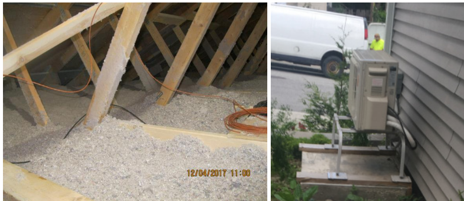
Figure 53. Insulated attic; heat pump outdoor unit
