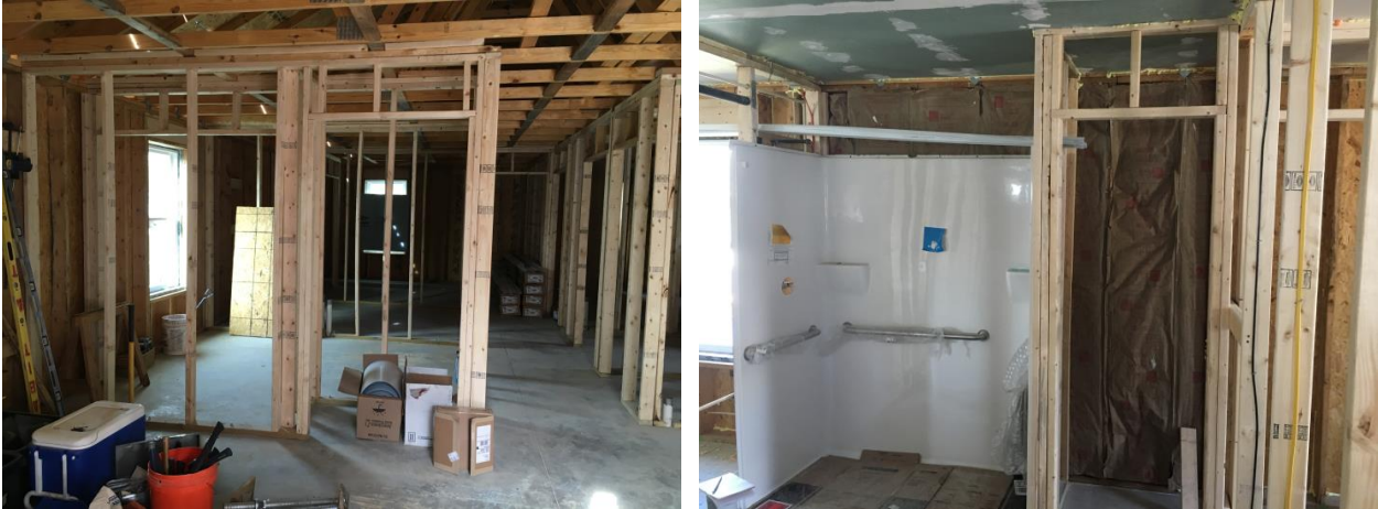
Figure 65. Maryland home interior rough framing (left); sealed ceiling plane and insulated walls (right)
