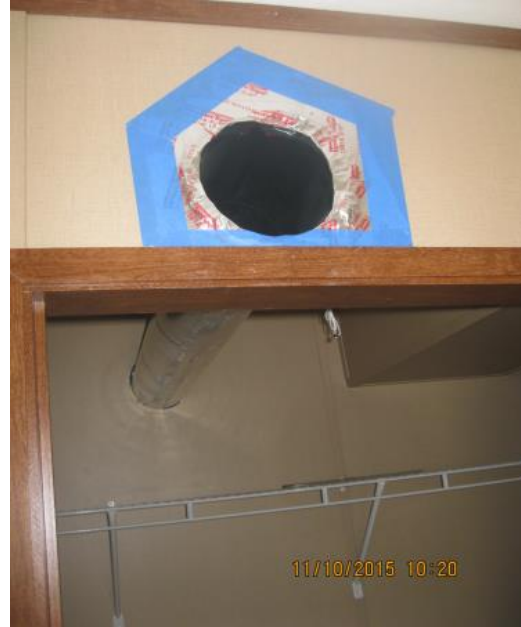
Figure 8. Master bedroom transfer fan bedroom side showing duct through closet (air outlet)
