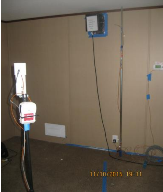
Figure 7. Master bedroom transfer fan at the living room side (air inlet)
