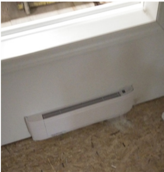
Figure C-32. Electric resistance backup heater installed in bedroom
