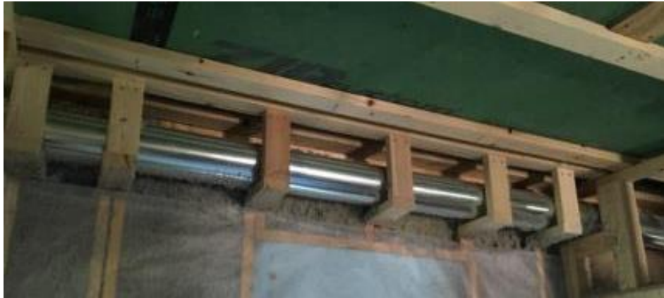
Figure 52. Transfer fan duct; an air barrier enclosed the cellulose within the wall cavity and drywall covered the soffit
