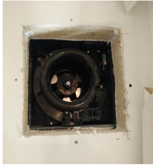
Figure C-31. Transfer fan viewed from bedroom closet
