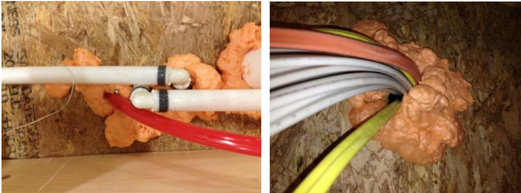
Figure C-3. Expanding foam with air gaps at floor decking penetrations
