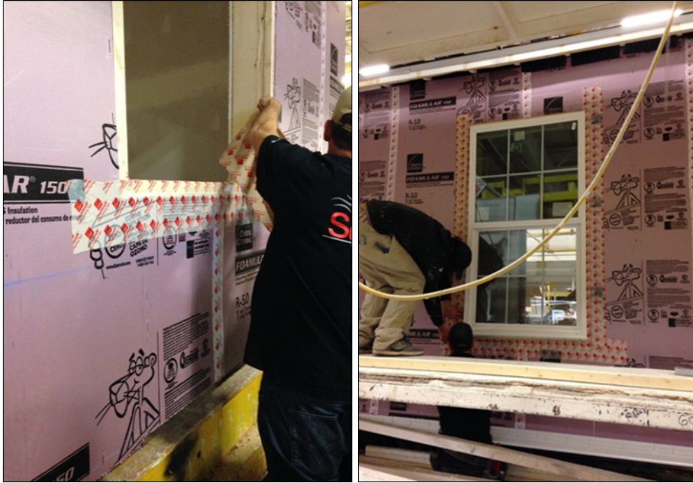
Figure C-23. Owens Corning representatives trained plant employees on airtight window flashing installation with Owens Corning FlashSealIR Tape
