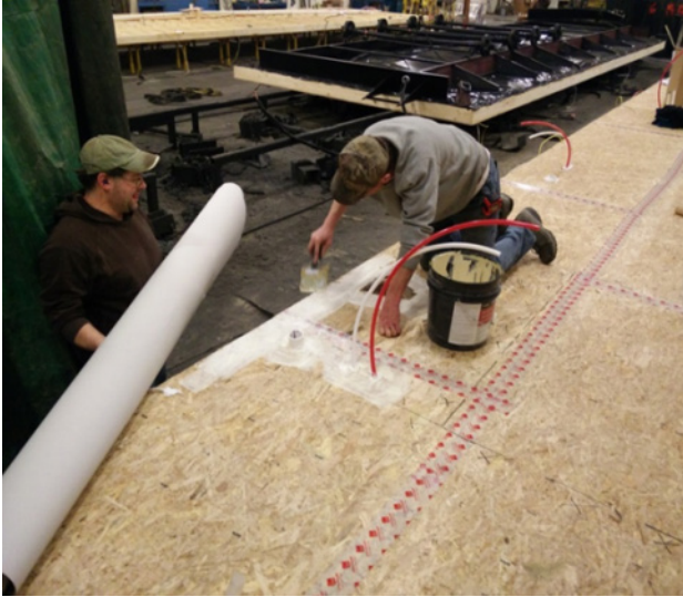
Figure C-13. Applying adhesive to edge of bathroom footprint receiving vinyl flooring; note air-sealing tape at OSB floor deck seams
