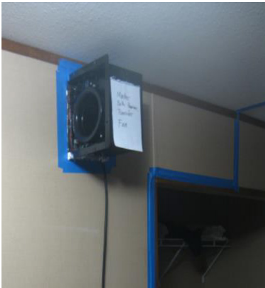
Figure 5. Transfer fan serving the master bathroom shown from the dining room side (air inlet)
