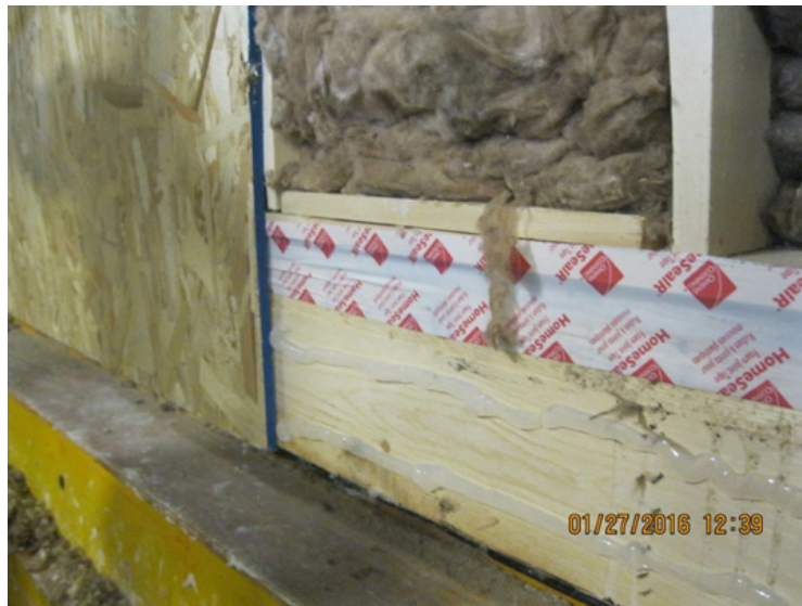
Figure C-21. Floor-wall joint sealed with tape; two beads of silicone caulk seal OSB wall sheathing to rim joist
