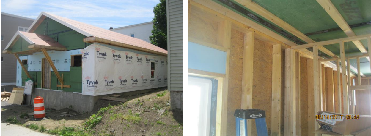
Figure 49. Framing outside (left), inside (right) showing OSB ceiling air barrier sealed with tape
