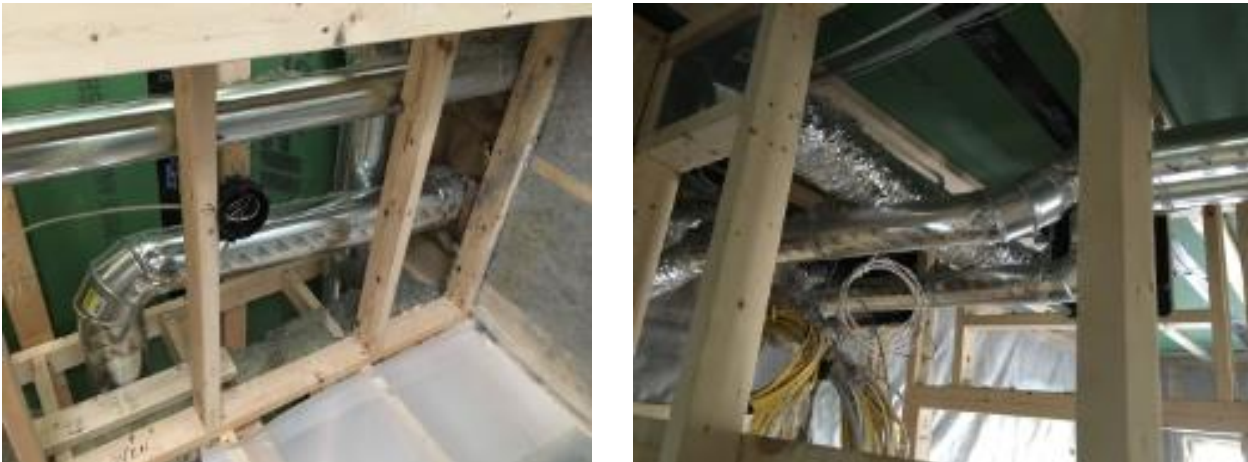
Figure 51. Ventilation and transfer fan ductwork
